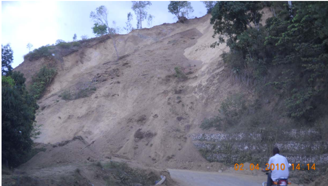
Figure 9.11 Relatively shallow slip-out of regolith. Disaggregated material flowed over stable gabions and blocked over half the road. (N 18.409159, W72.638815).
