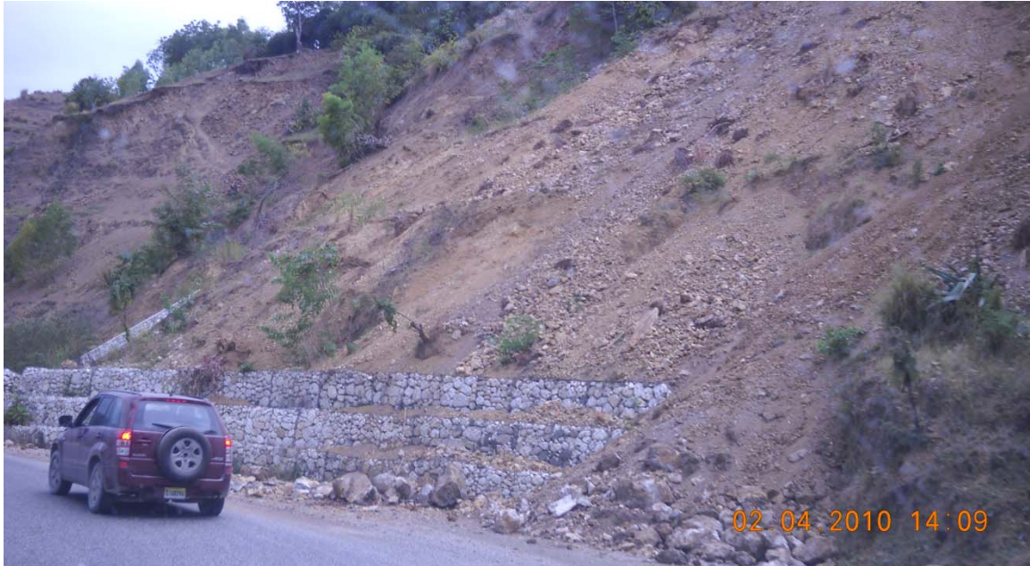
Figure 9.10 Shallow rock topple or rock fall from over-steepened road cut. Debris slid over the top of stable gabions at the toe of the slope. (N18.409159, W72.638815).
