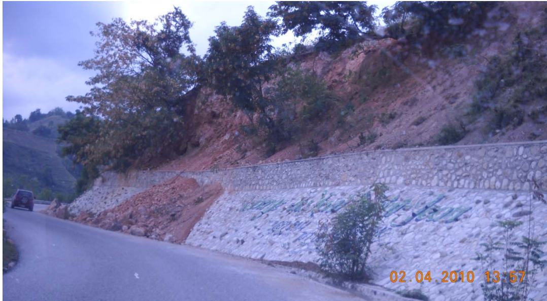
Figure 9.12 Shallow slip-out of soil in upper road cut. Soil slid over the top of the surviving masonry wall and slope protection. (N18.440270, W72.636207).
