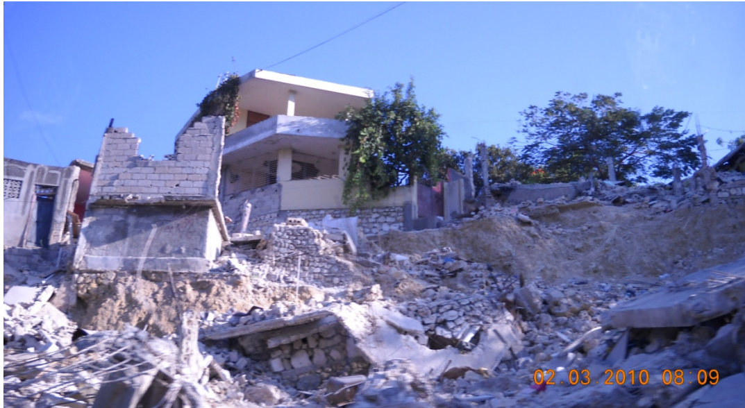
Figure 9.7 Several buildings have collapsed in this location. Although there are scarp-like near vertical surfaces near the top of slope that may suggest the possibility of a deeper rotation failure, in our opinion the observed conditions are likely due movement of soils adjacent to failed walls, as discussed in the text. (N18.528406, W72.309920).
