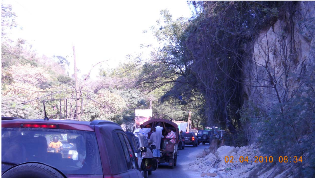
Figure 9.5 Vertical cut remaining relatively stable with minor rock fall/topples.
